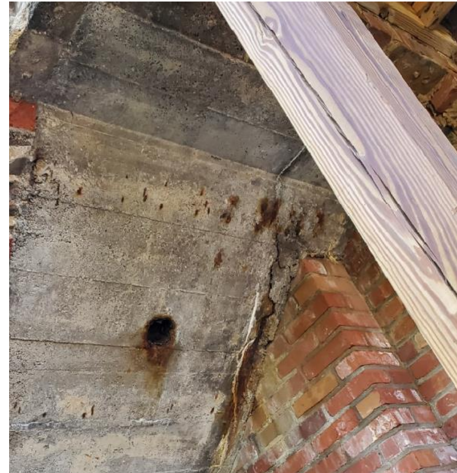
Cracking in Underside of Staircase
