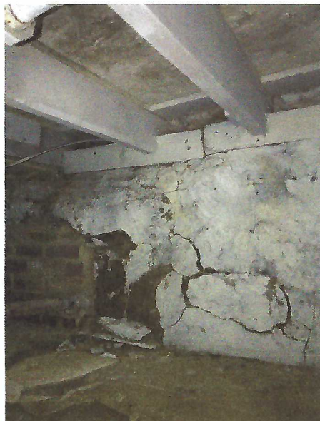
Deterioration of north foundation wall and notched floor joists.
