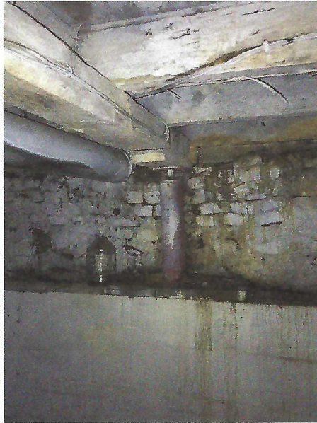
Deterioration of west foundation wall also showing beam and joist members.
