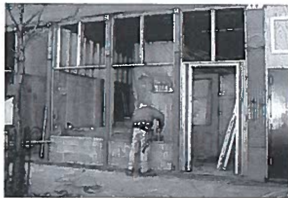
Floodproofing the vestibule of a storefront
