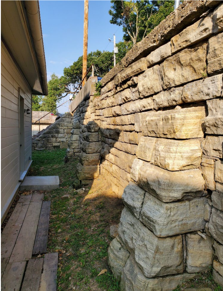
Limestone Retaining Wall Structurally Failed
