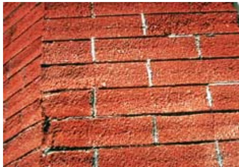
Historic brick damaged by sandblasting.
