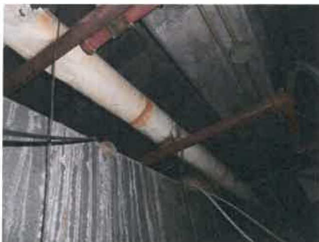
Sample location 1-PW3 (Asbestos Present)
