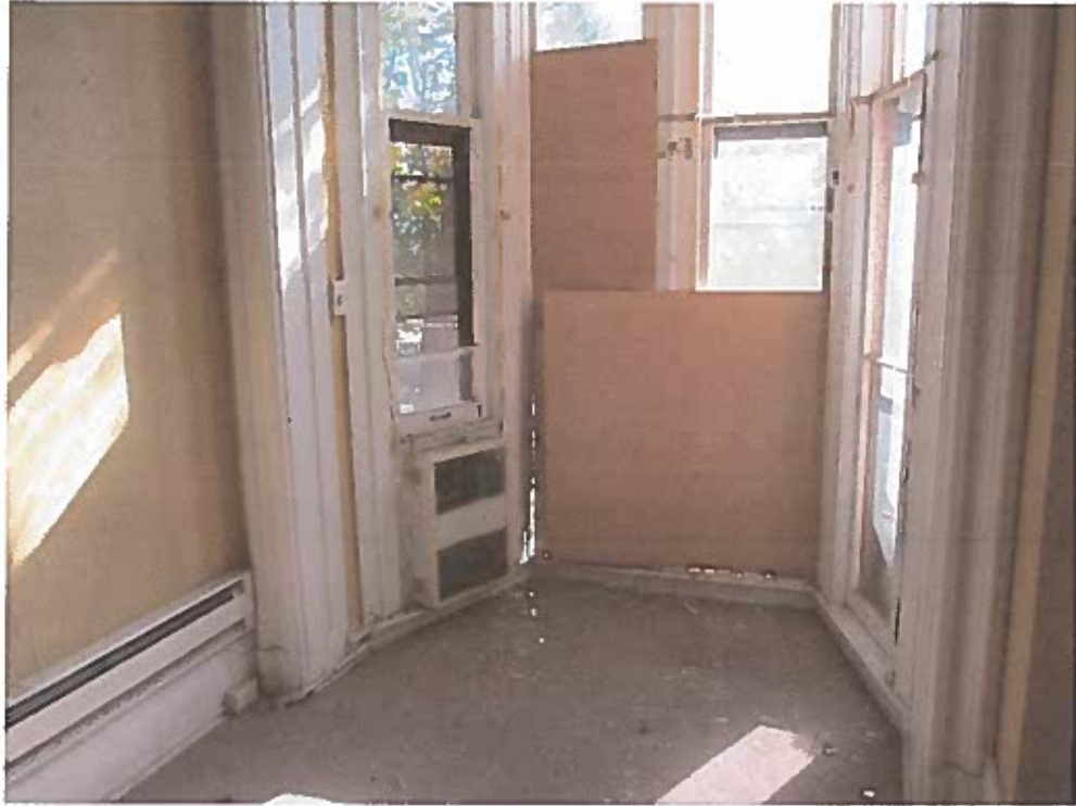
First Floor – Damaged windows
