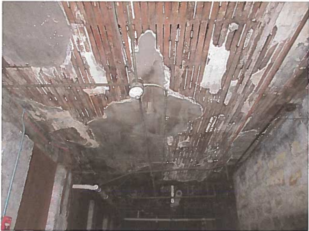
Basement – Damaged ceiling
