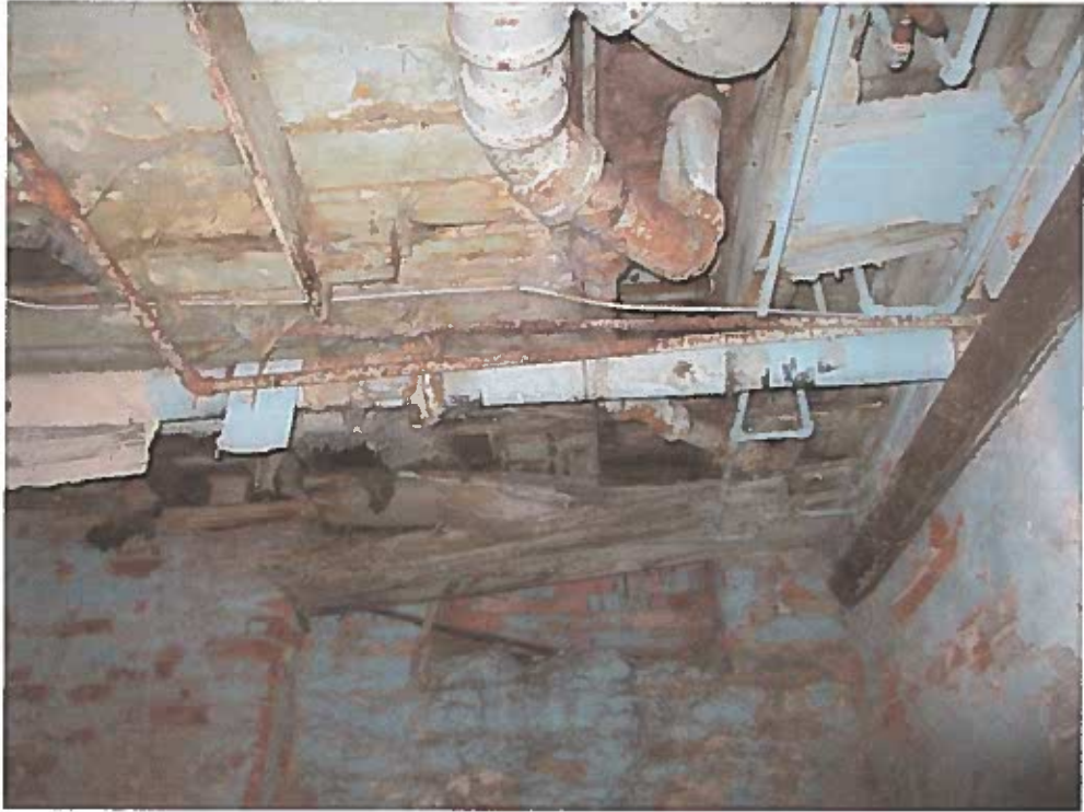
Basement – Damaged ceiling
