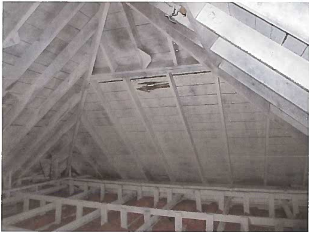
Third Floor – Dormer framing with damaged sheathing
