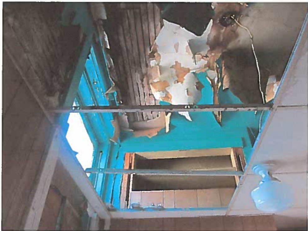
First Floor – Water damage ceiling and exterior wall
