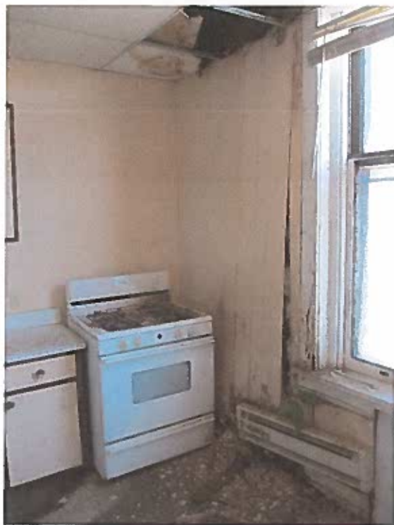
Second Floor – Water damage at exterior wall
