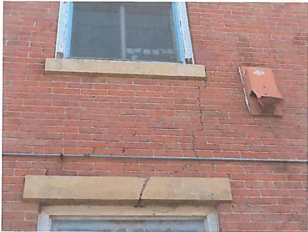
Exterior – Cracking at stone lintel & brick masonry
