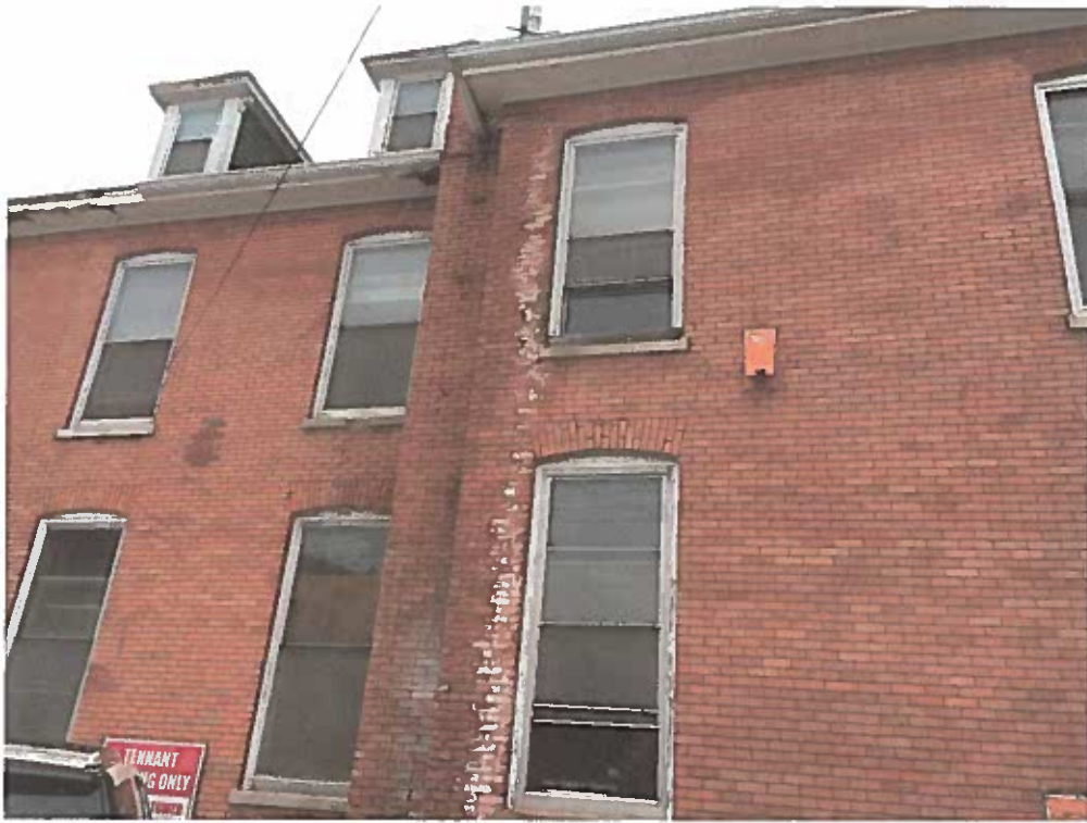
Delaminated and Saturated Brick / Rotted Roof Overhang
