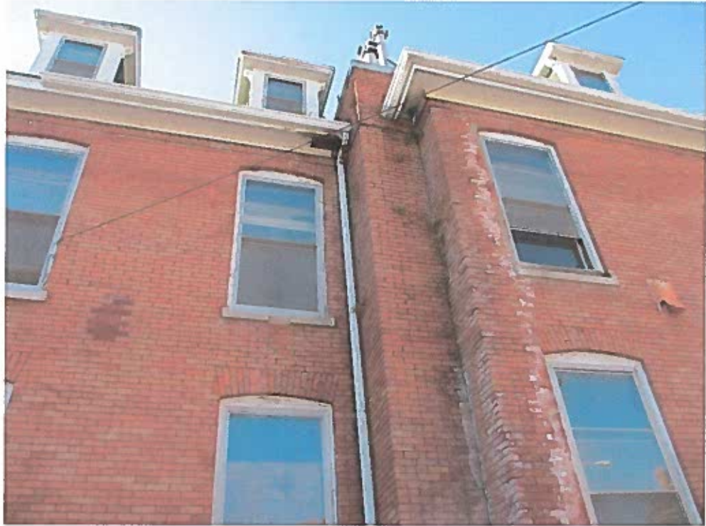
Exterior – Water damage at brick and soffit
