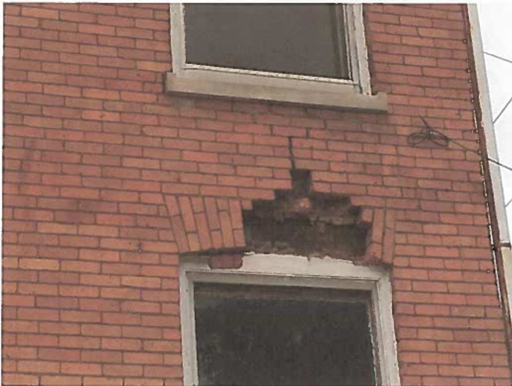
Missing Brick / Rotted Windows
