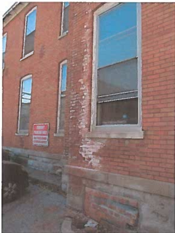
Exterior – Water damage at brick
