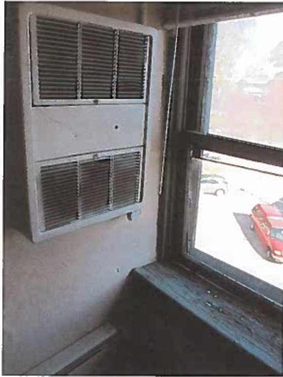
Third Floor – Deteriorated window sash and window sill
