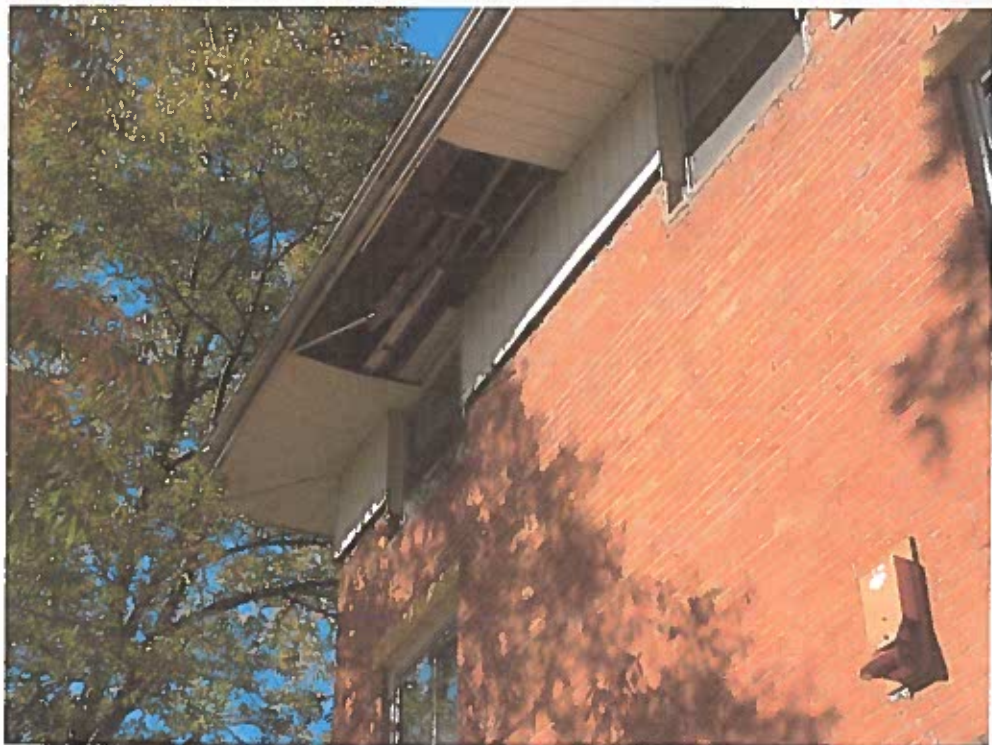
Exterior – Missing soffit
