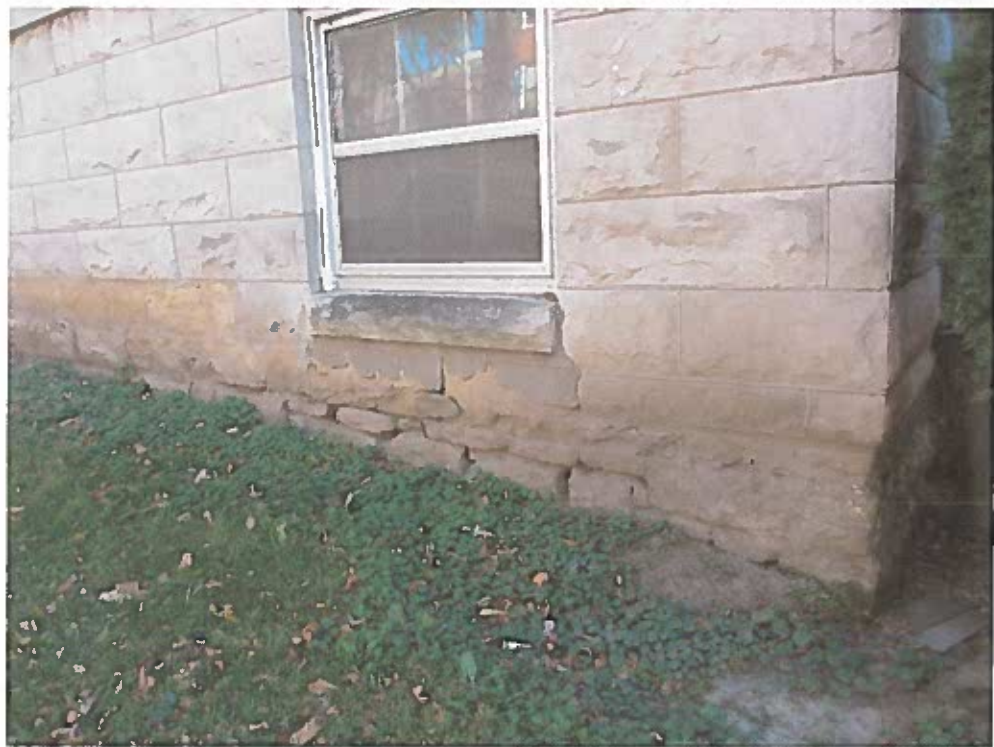
Exterior – Eroded joints at stone foundation
