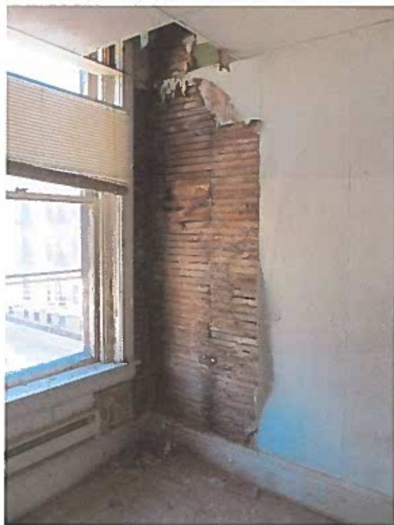
Second Floor – Water damage at exterior wall
