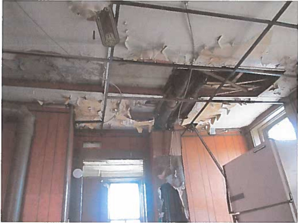
First Floor – Water damage at ceiling
