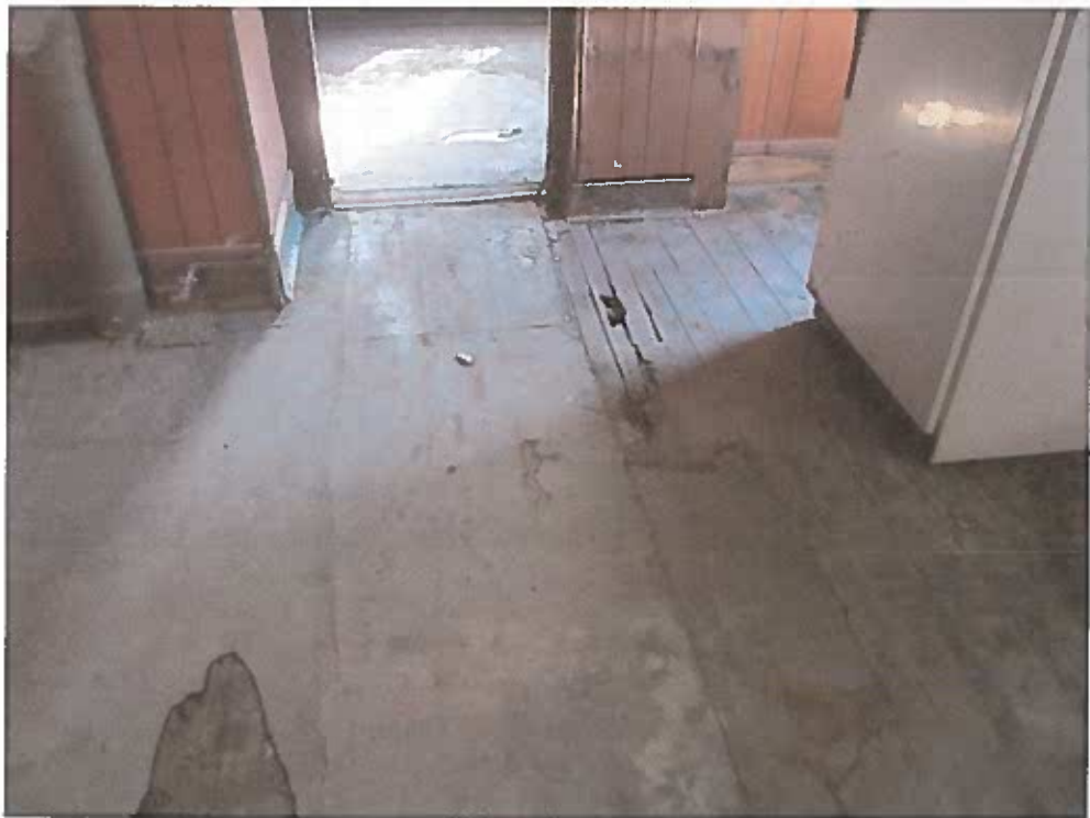
First Floor – Water damage at floor
