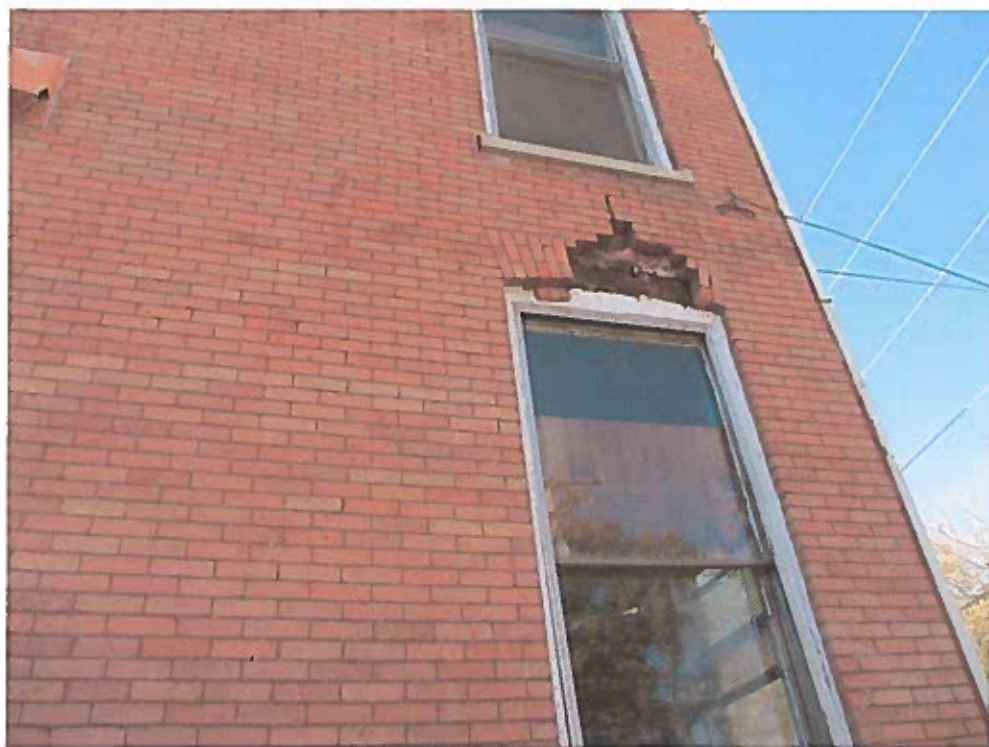
Exterior – Missing brick
