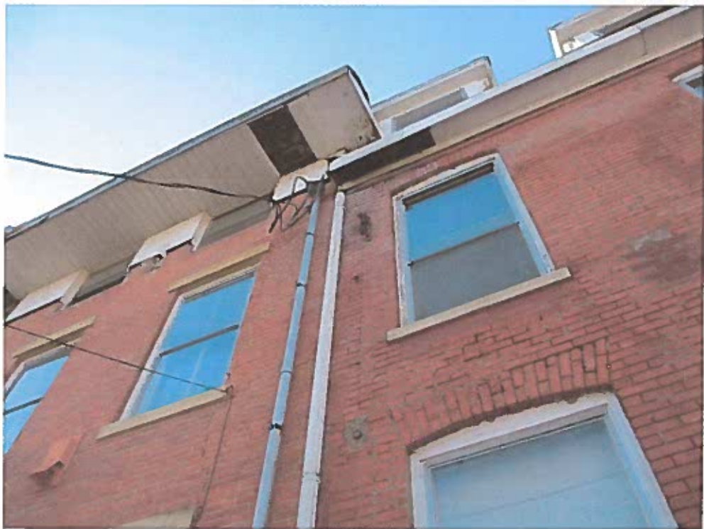
Exterior – Missing soffit
