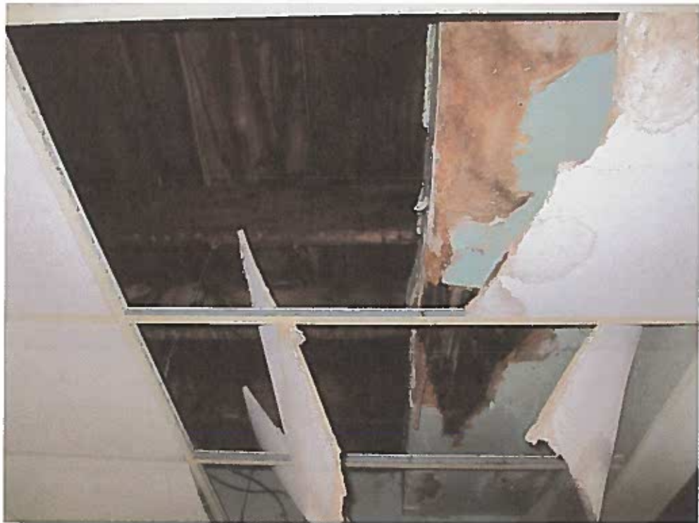
Third Floor – Missing plaster at cupola floor framing
