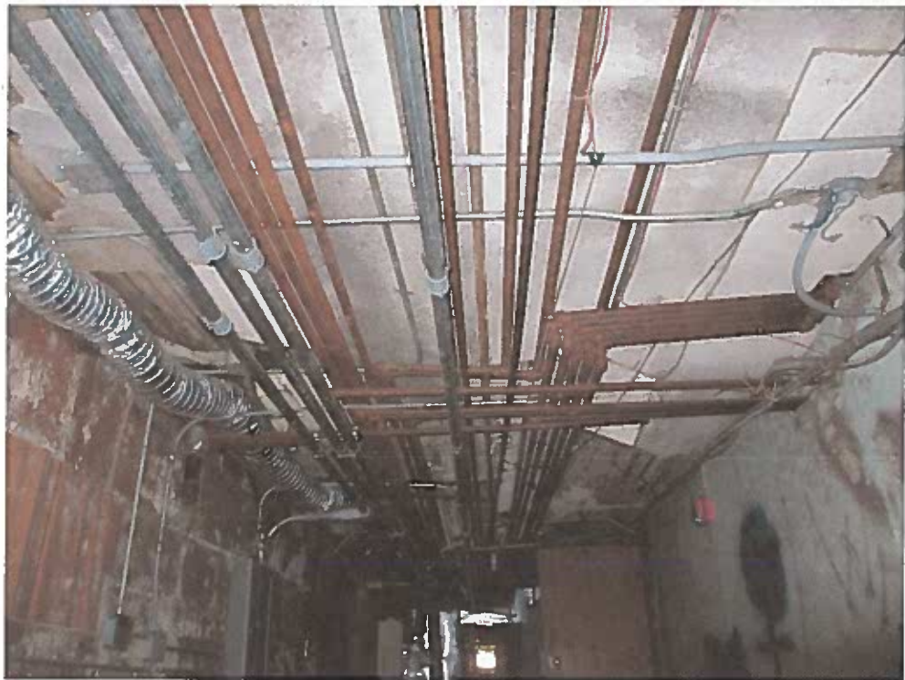
Basement – Piping & conduit at corridor ceiling
