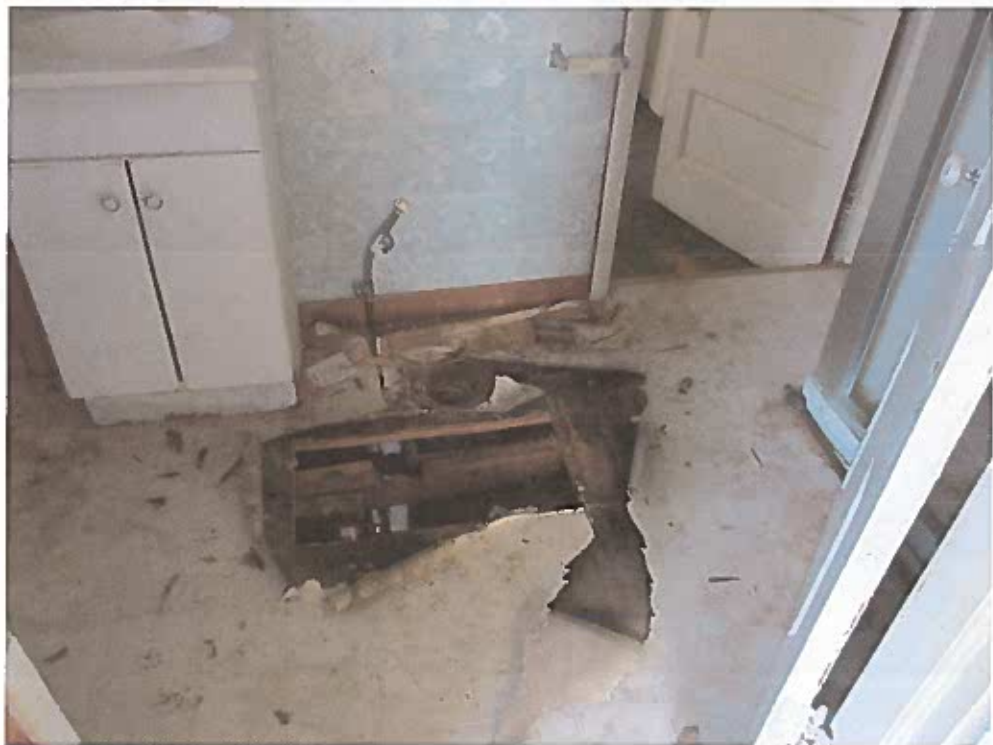
Second Floor – Damaged floor
