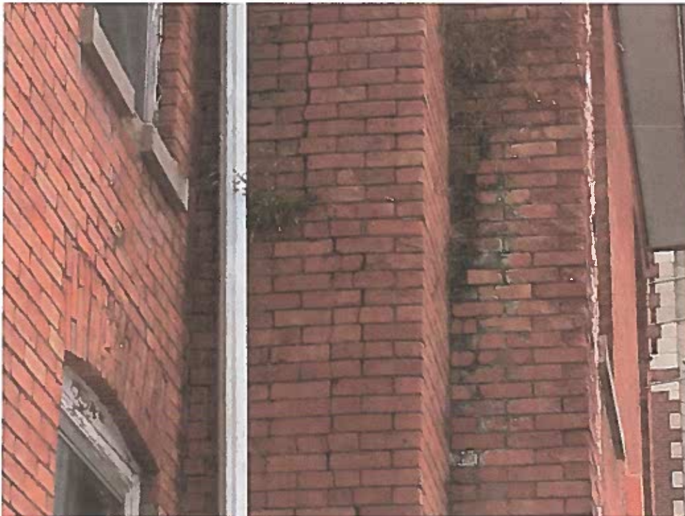
Cracked and Delaminated Brick
