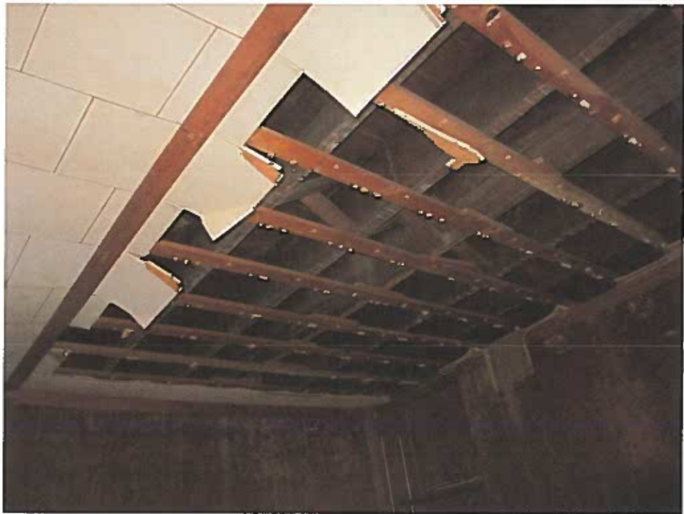
Basement – Damaged ceiling
