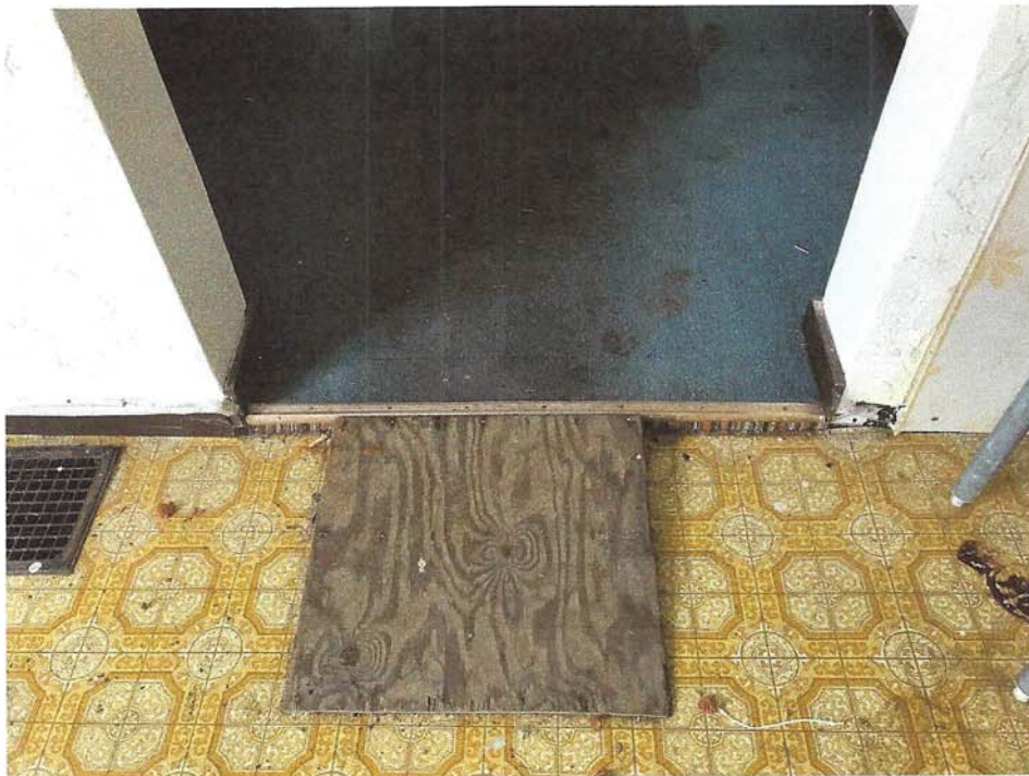
8. Approximate 2-inch floor elevation difference between rooms.
