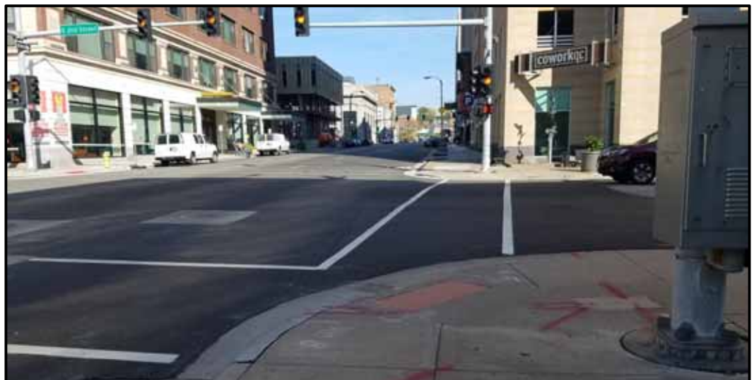
Figure 15. Misaligned Crosswalk due to Corner Ramp.
