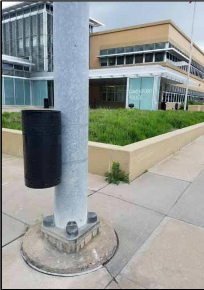
Figure 27. Trash Receptacle on Utility Pole.
