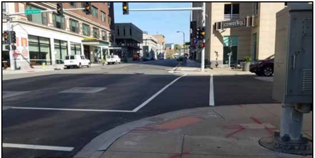
Figure 14. Misaligned Crosswalk due to Corner Ramp.
