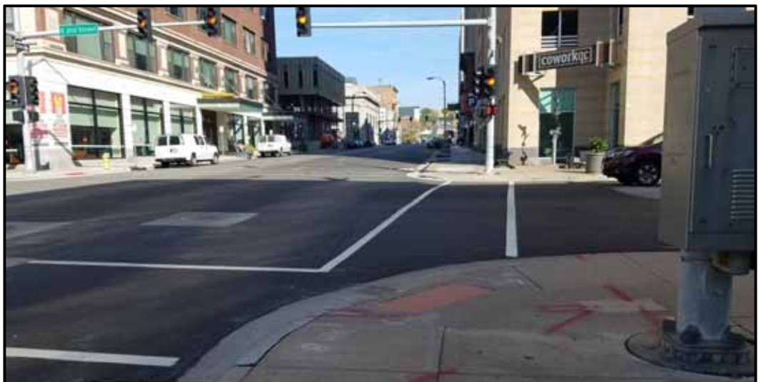
Figure 14. Misaligned Crosswalk due to Corner Ramp.
