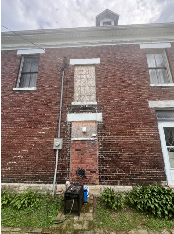
Exterior view of boarded window from alley
